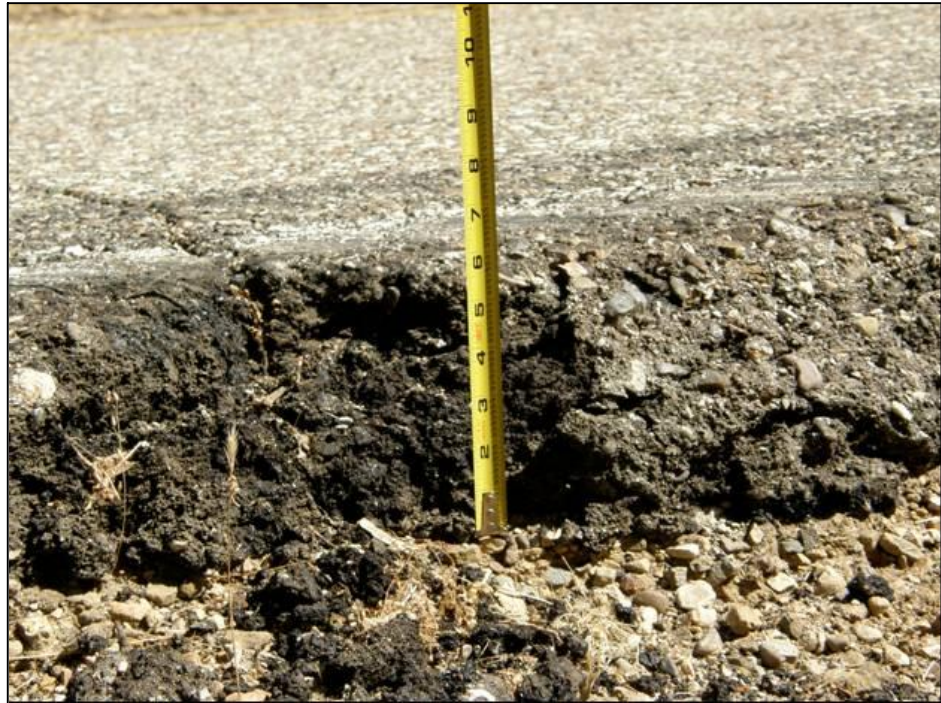
Fig 3 – Asphalt thickness and road edge where Engine 56's rear dual tires went off Vasquez Road.
